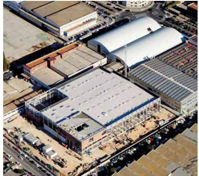
Aerial view of the building works of what will become the online purchasing distribution centre in the Vara de Quart industrial estate in Valencia.
